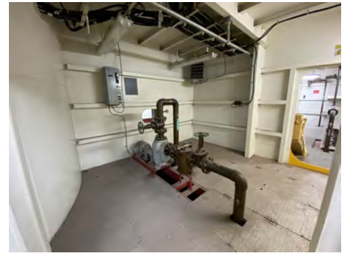
Aft Machinery/Pump Room Cont.
