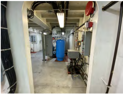
Freshwater Pump & Heater
