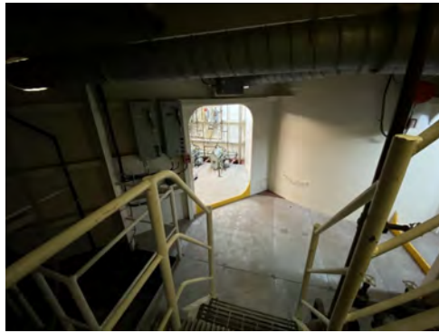
Aft Machinery/Pump Room
